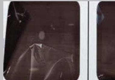
Self-applied sun protection or tinted strips must be completely removed from the glass area if they have not been professionally applied, are torn, or have begun to peel away at the corners.
